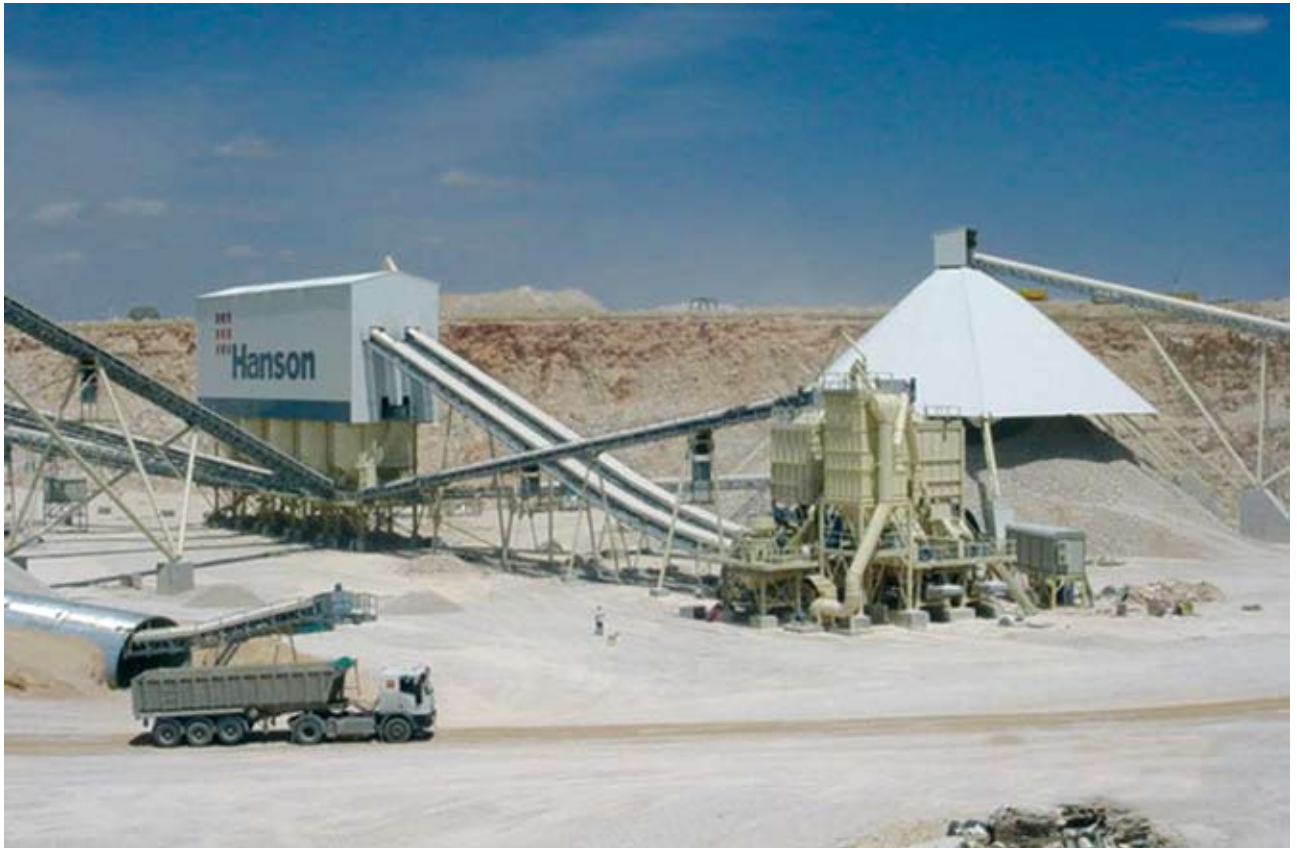
Valdilecha Plant, Hanson Group: a newly erected complete crushing and screening plant for producing multiple end products of limestone near Madrid, Spain .
