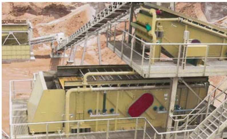
Plant with Nordberg Gfa vibrating equipment.
